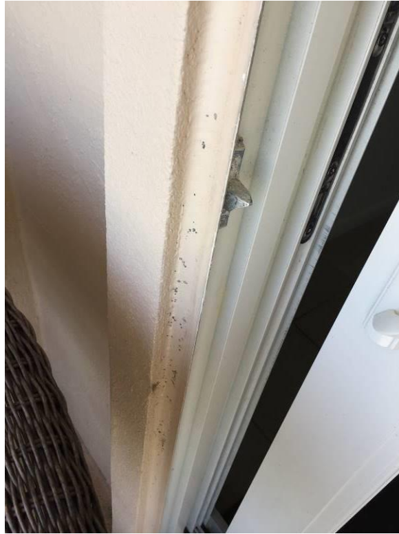
Photograph #17 – Black spotting through sliding glass door perimeter sealant
