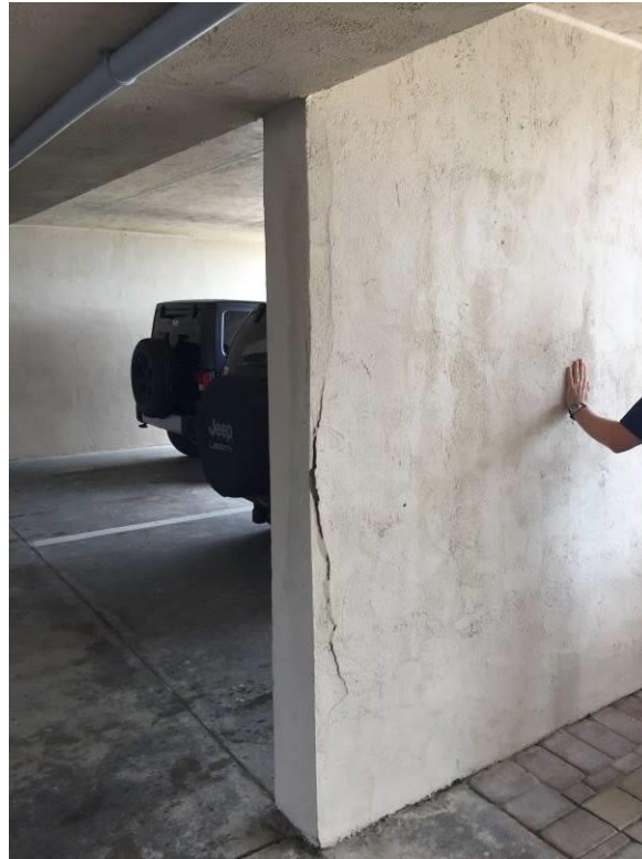
Photograph #3 – Typical spall on load bearing wall in ground floor parking area
