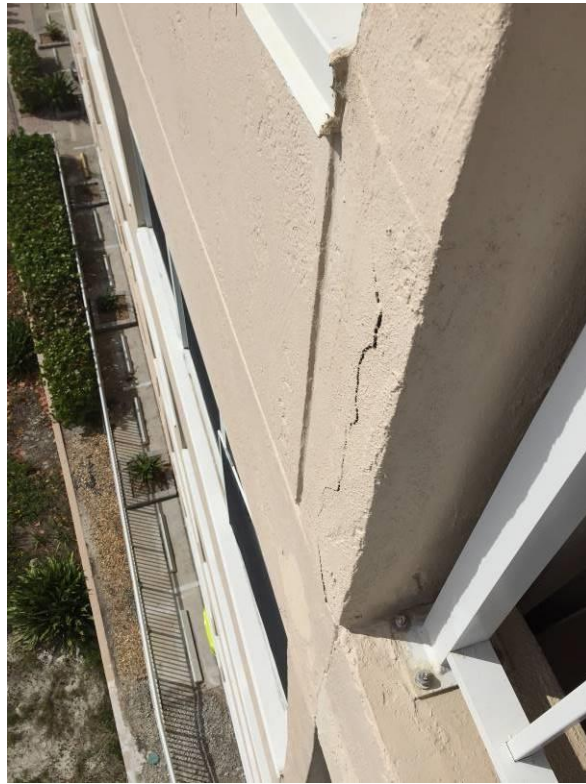
Photograph #7 – Cracking in framed wall between the balcony and window
