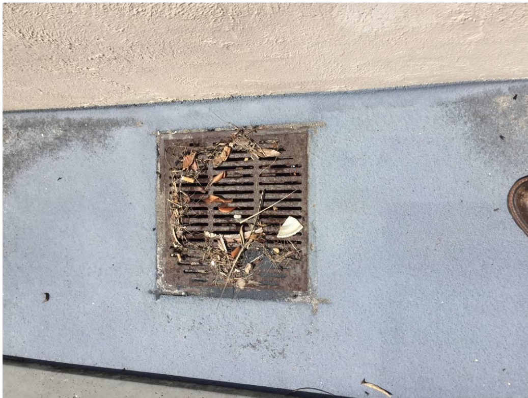
Photograph #28 – Typical corroding parking structure drain
