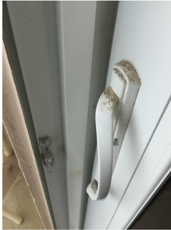
Photograph #23 – Typical oxidizing sliding glass door hardware
