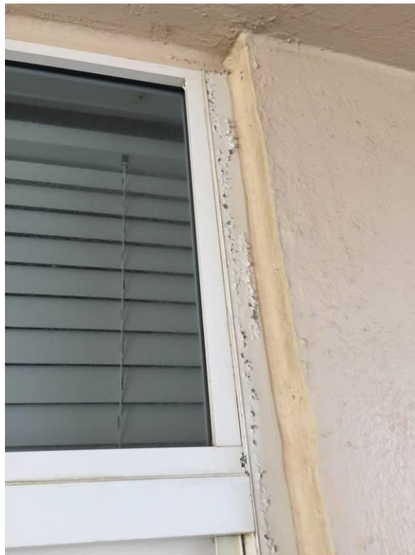
Photograph #26 – Typical oxidizing window
