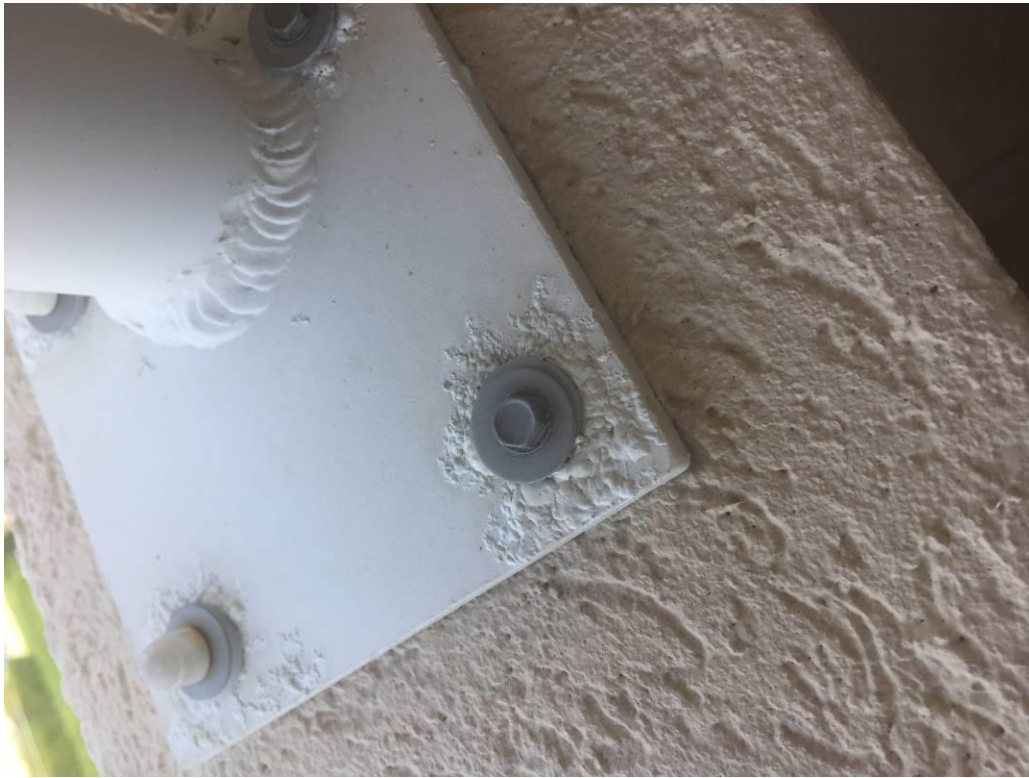
Photograph #21 – Typical oxidation on walkway guardrail base plates
