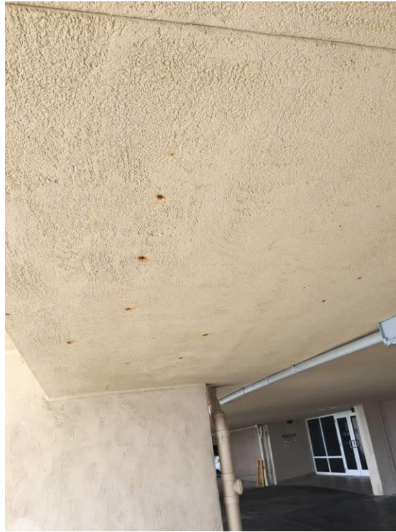
Photograph #29 – Typical rust spots on drop down soffit of ground floor parking area
