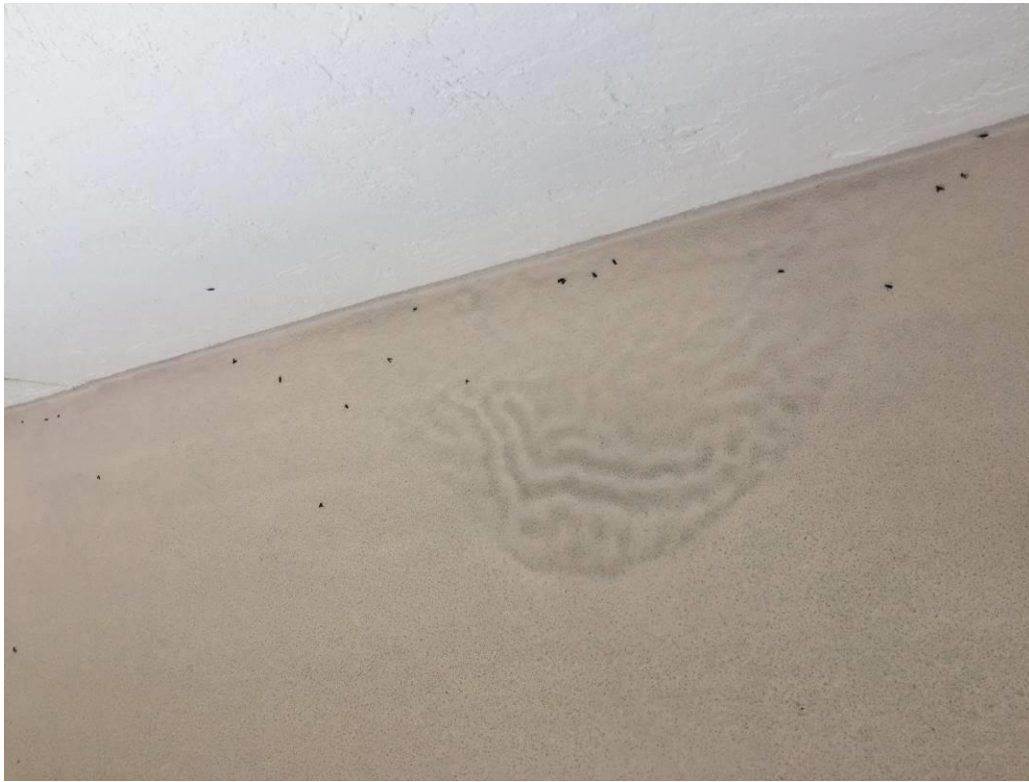
Photograph #13 – Wrinkles in walkway deck coating
