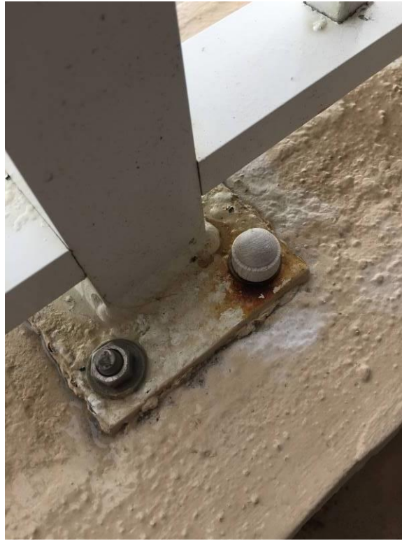
Photograph #19 – Typical balcony guardrail base plate with oxidation and rust bleed
