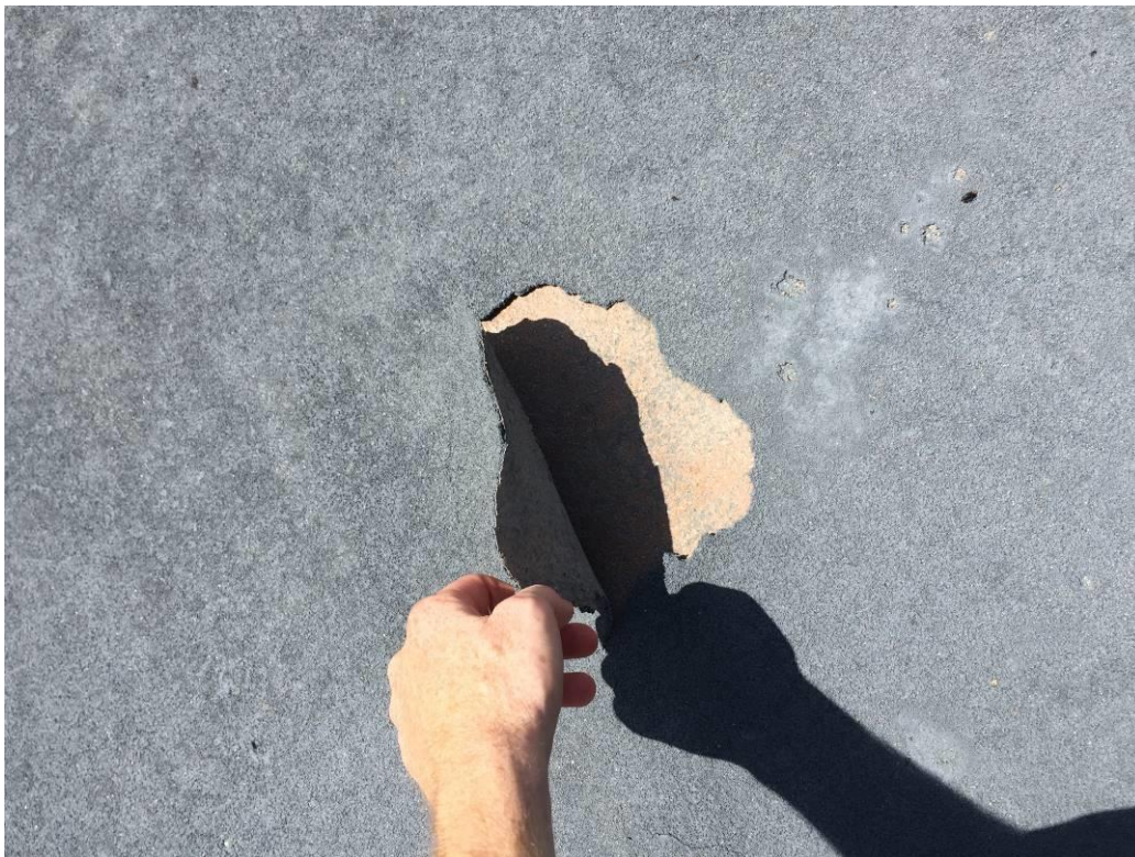
Photograph #14 – Failed deck coating on parking structure
