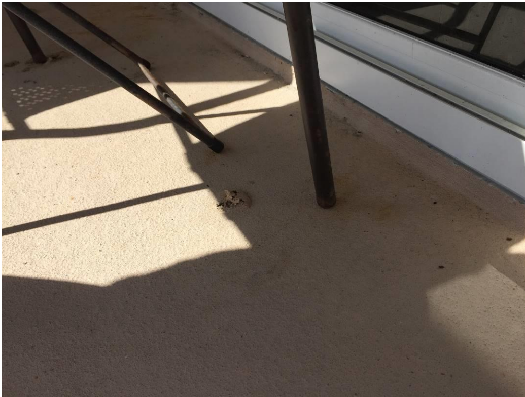
Photograph #11 – Deck coating failure on balcony
