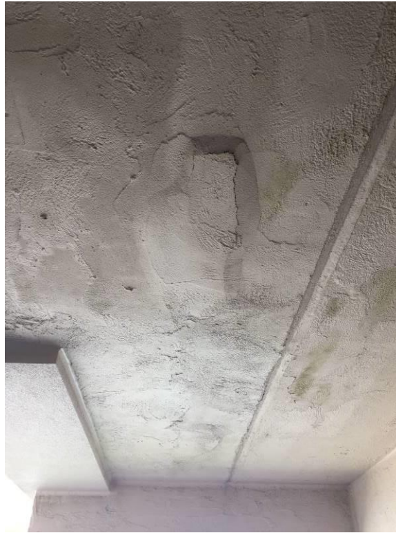
Photograph #1 – Typical ceiling spall on walkways
