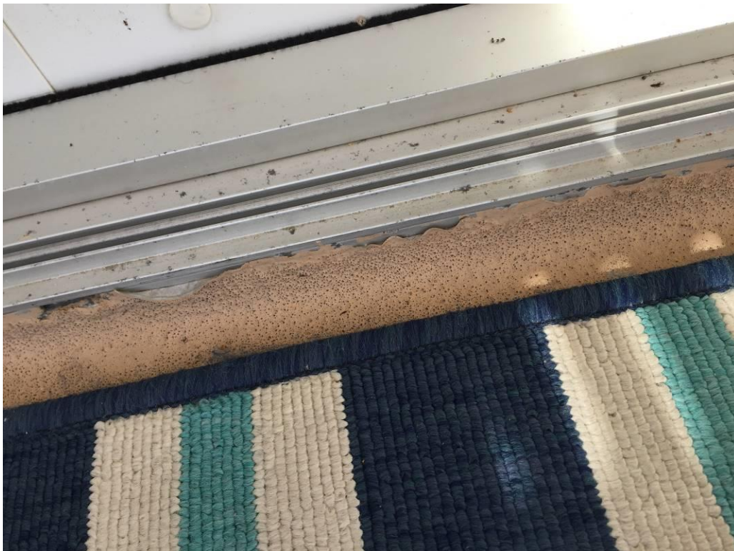
Photograph #24 – Typical oxidizing sliding glass door threshold with failed coating
