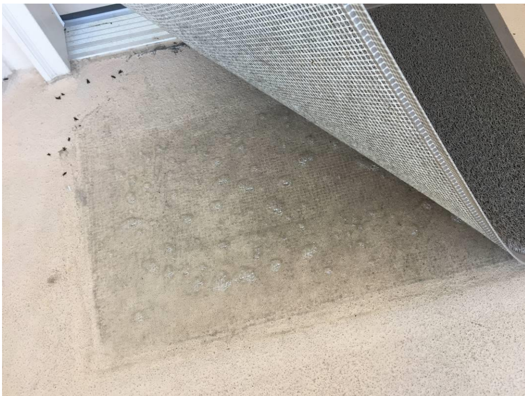
Photograph #12 – Water being held under unit entry door mat
