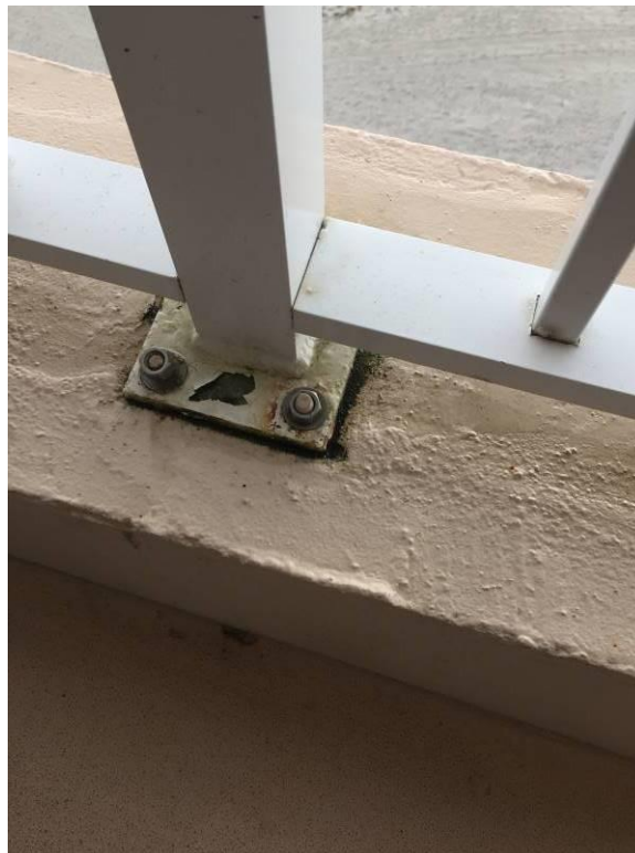
Photograph #20 – Typical flaking paint on balcony guardrails
