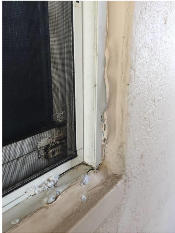
Photograph #25 – Typical oxidizing window
