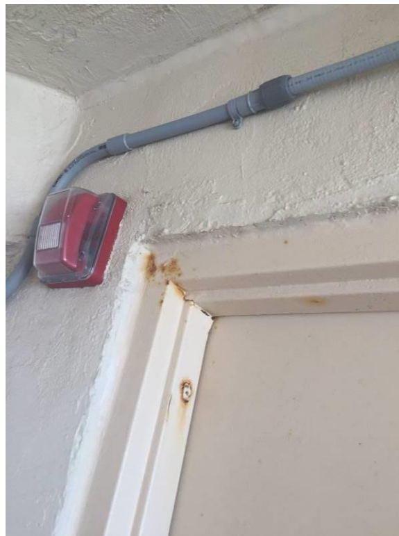
Photograph #8 – Typical corrosion of common walkway door frames
