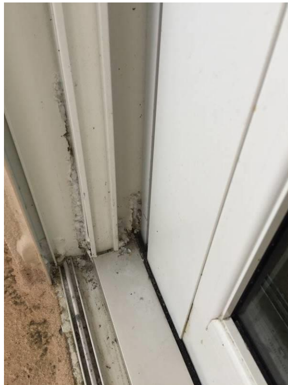
Photograph #22 – Oxidizing sliding glass door framing
