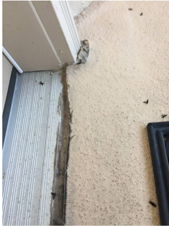
Photograph #27 – Unit door with topping higher than threshold
