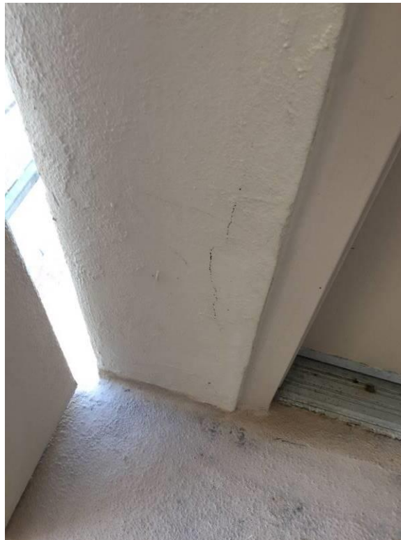
Photograph #2 – Typical jamb spall on stairwell door
