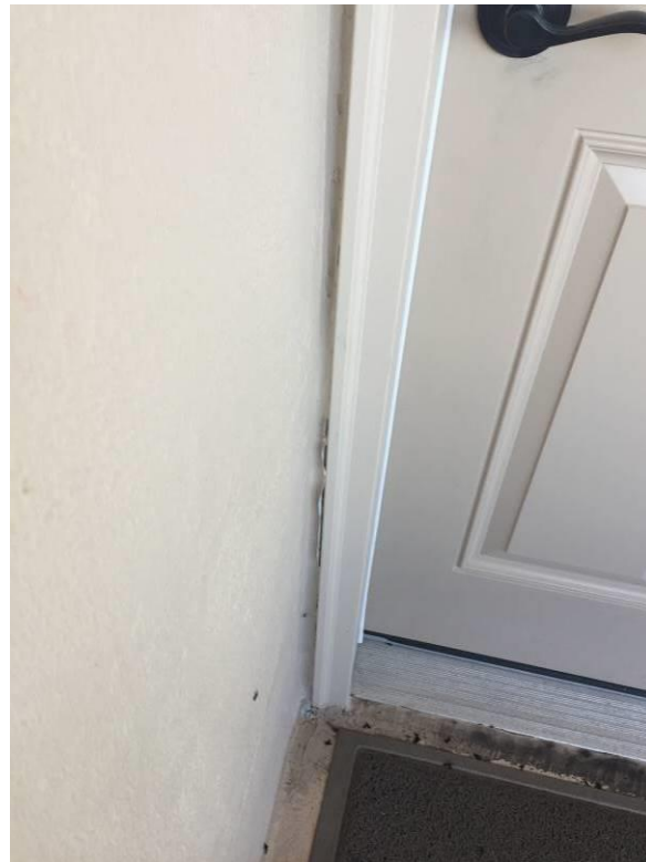
Photograph #16 – Failed perimeter sealant at unit entry door
