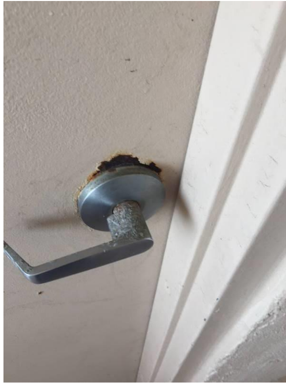
Photograph #9 – Typical corrosion on walkway common door slabs
