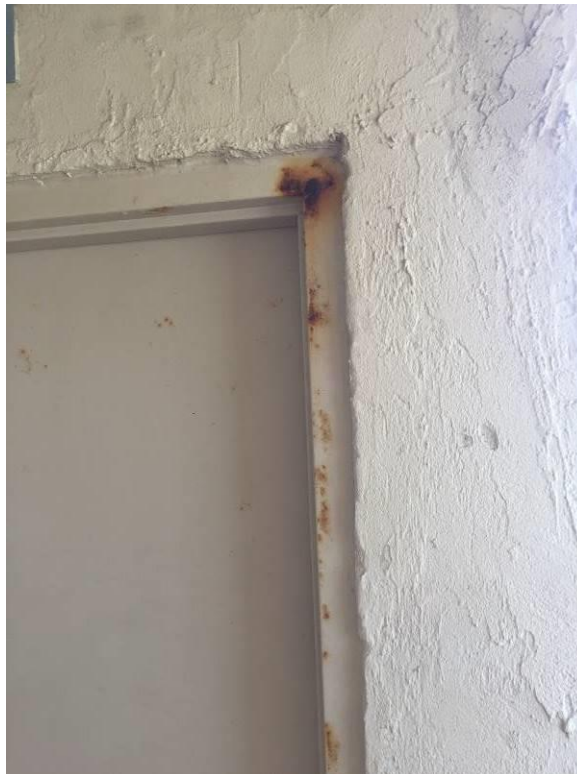
Photograph #10 – Typical corrosion on walkway common doors
