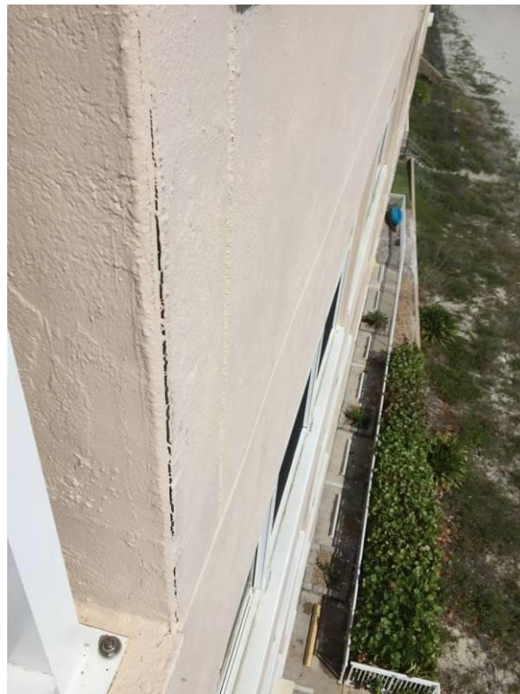
Photograph #6 – Typical cracking on framed wall section between balcony and window
