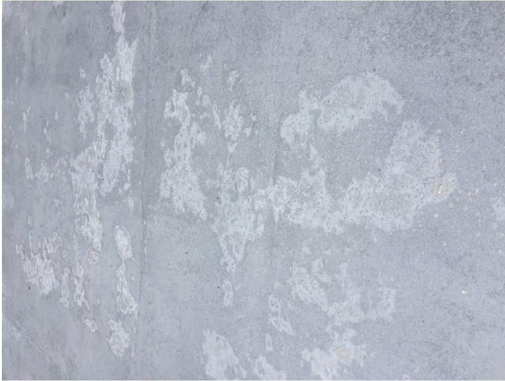
Photograph #15 – Failed deck coating on parking structure
