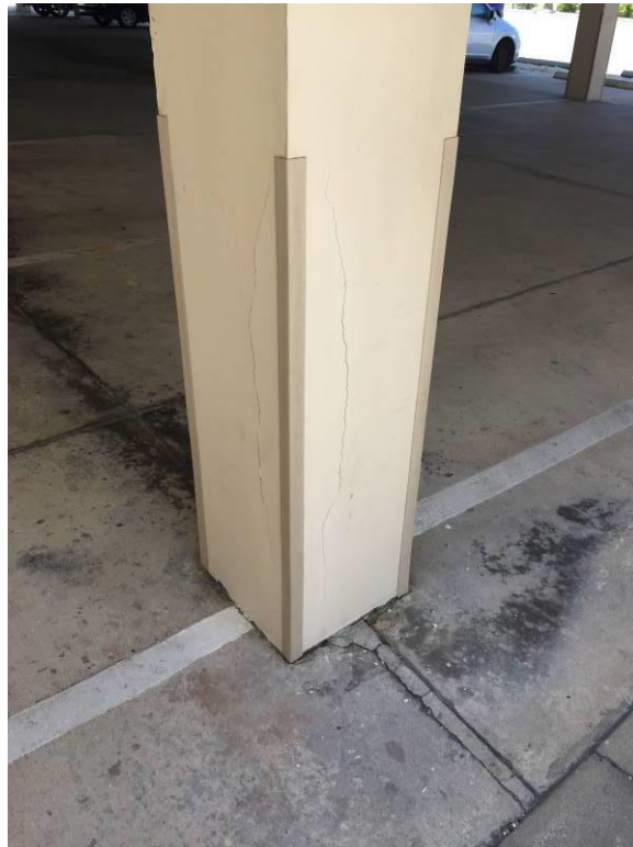
Photograph #5 – Typical column spalling on parking structure
