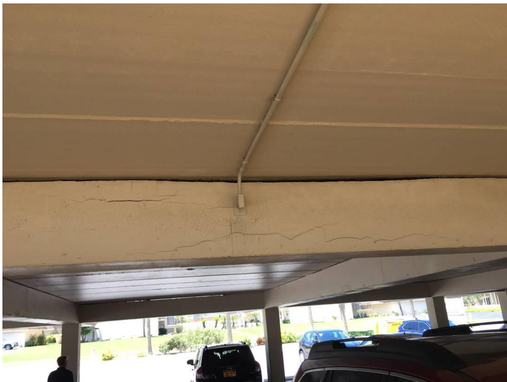
Photograph #4 – Typical spalling on beams supporting the parking structure
