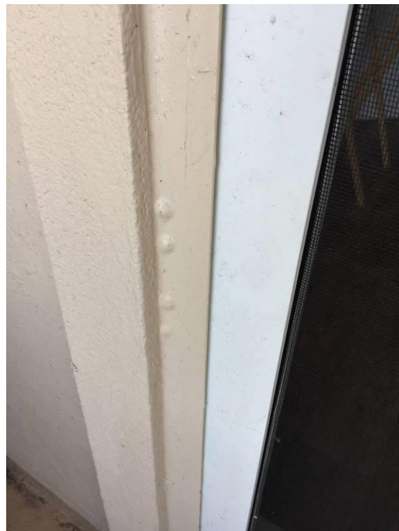
Photograph #18 – Blisters in perimeter sealant
